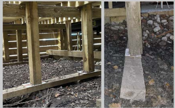
Some support posts appeared to be floating - unconnected to the uneven ground, there was a haphazard mix of timber joist off-cuts and non-durable plywood was being used as packing material.
