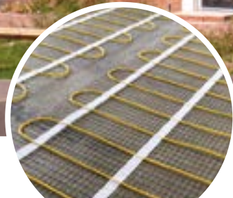
Electric 'dry' systems
