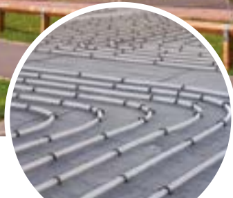
Hydronic 'wet' systems
