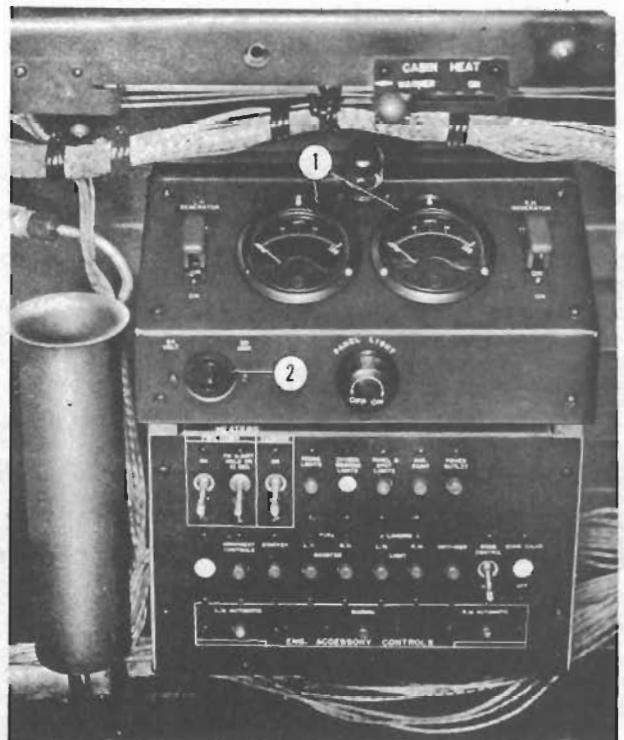
Figure 42A—Generator Control Panel (P-61B)
