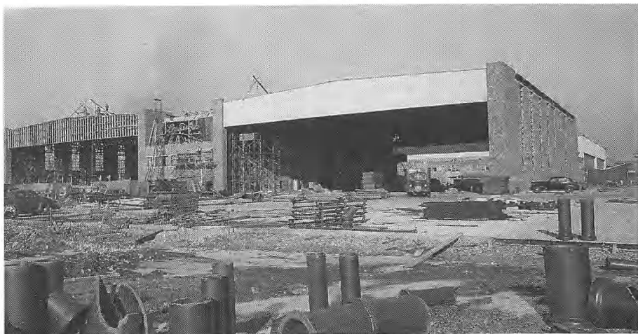
The size of the test hangar is apparent as the building nears completion. Photo courtesy of the Connecticut Air and Space Center, Stratford, CT.
